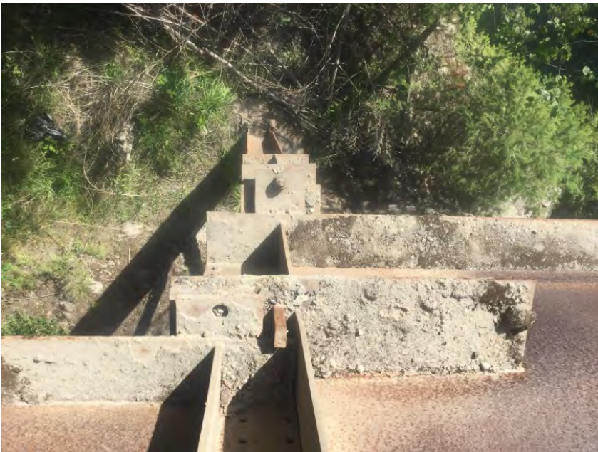
Left span to main span restrainers in place and functional
