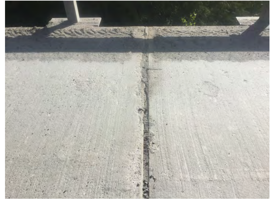
Main span to left seal in place and functional but separating
